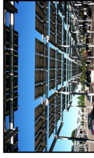
The world's largest parking lot solar system is located in Sacramento, California.
